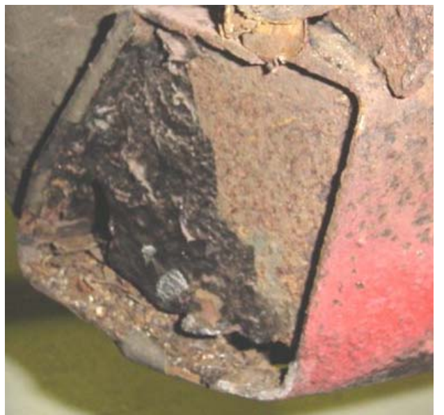
The frame end rails are rusted also.
