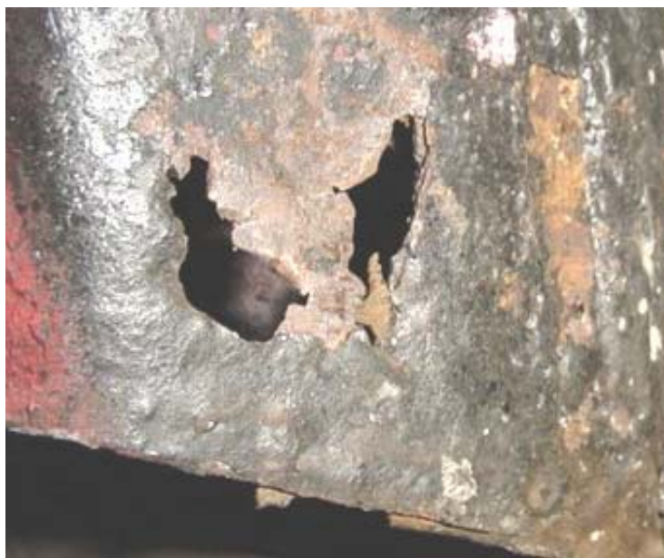
The frame was rusted through in places.
